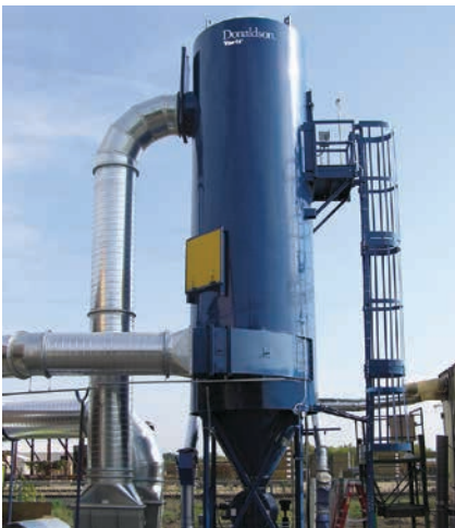
RF Dust Collector
